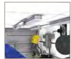
Full Electrical Service
